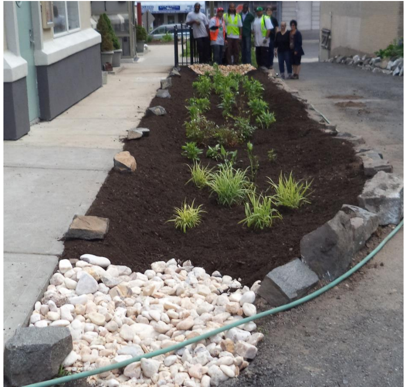
This 300 square foot rain garden captures church driveway rainwater runoff while beautifying the parking lot.
