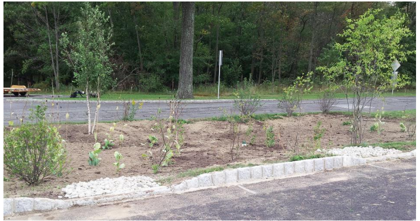
We can fix non-working rain gardens, too!
